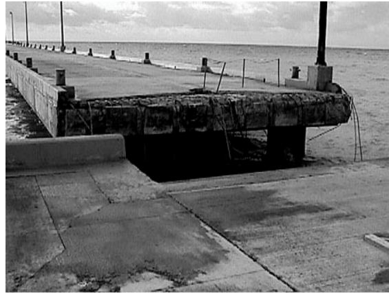
Damage to the Frederiksted pier.
