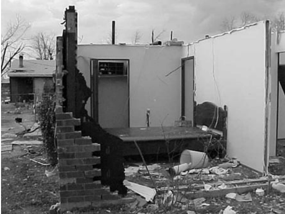
Owensboro, KY-- A waterbed is all that remains of this house that was directly in the path of a tornado that damaged more than 700 homes statewide.
