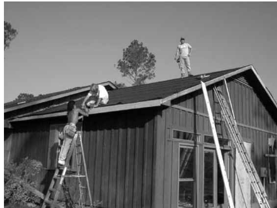
Camilla, Georgia -- Houses are being rebuilt and repaired here as residents recover from devastating tornadoes that struck on February 14th.
